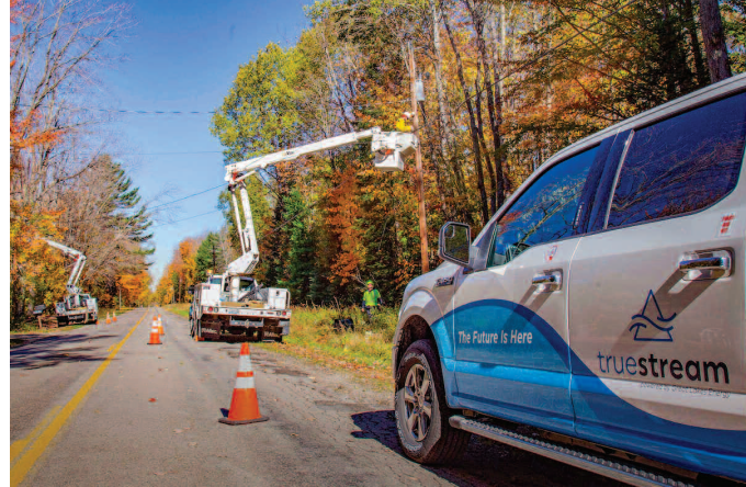
Great Lakes Energy has announced Phase I construction plans for its fiber network starting this spring in parts of its Boyne service area, which primarily covers rural areas in Charlevoix and Antrim counties. Courtesy photo
